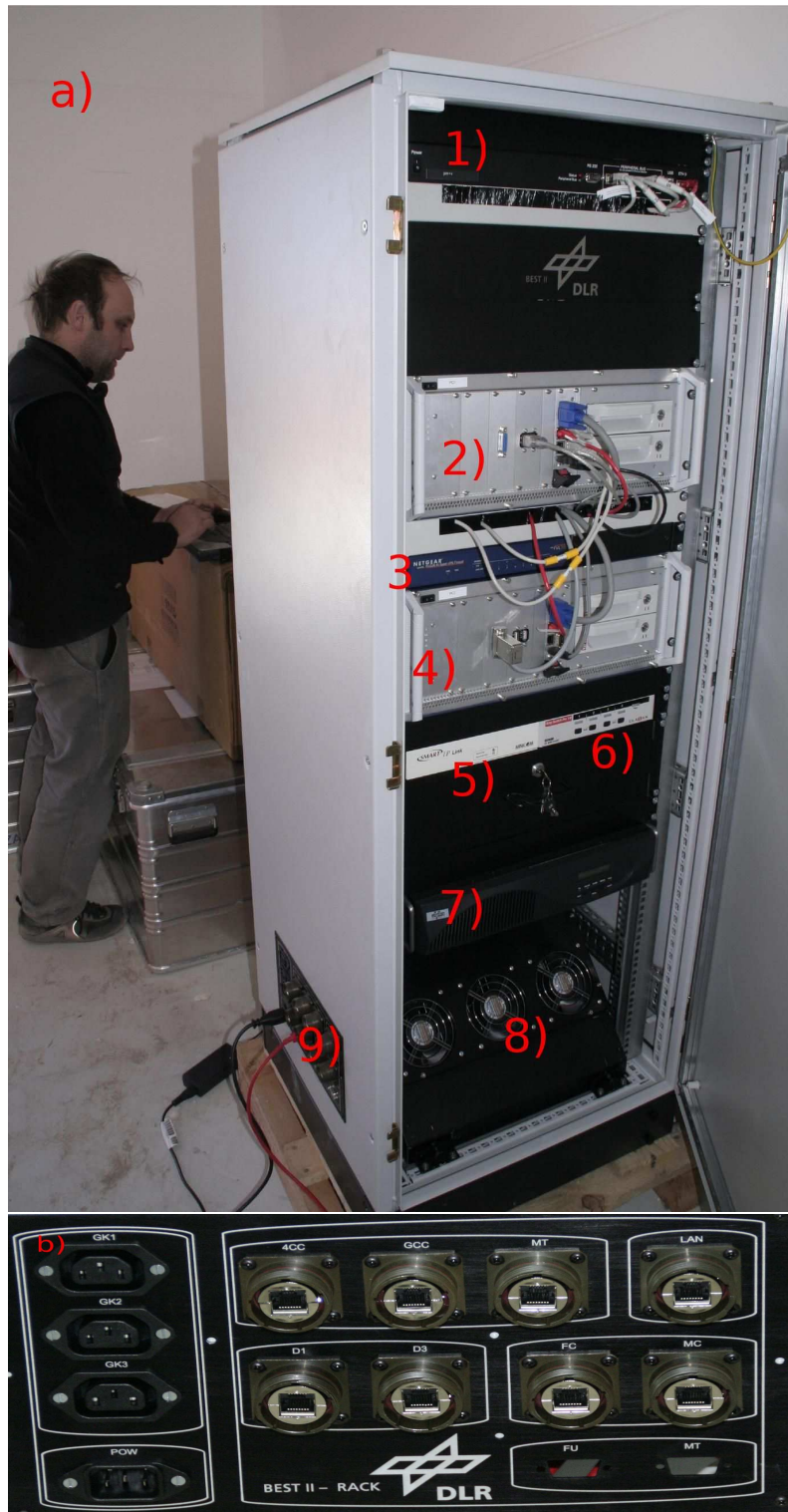
Figure 6.11: Figure a) presents the RACK with electronics controlling the system operations. 1) is the security master, 2) is PC1, 3) router, 4) PC2, 5) IP-link, 6) KVM-switch 7) battery, 8) fan, 9) interface with cable ports. Figure b) presents an interface for cables (see 9) in Figure a)) connecting the instruments with the control PCs. Ports: GK and POW - power supply ports, 4CC - scientific CCD, GCC - guider CCD, MT - mount, LAN - free port for LAN connection, D1, D2 - Internet ports, FC, MC - free ports.
