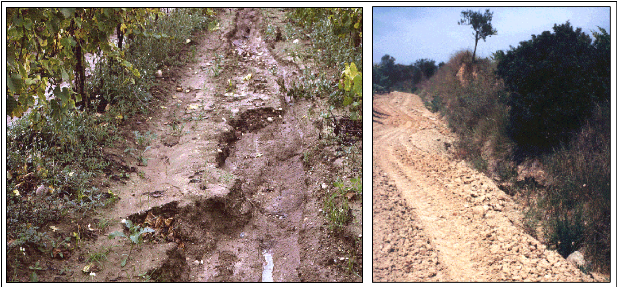
Figure 4.23. Left: ephemeral gully formed during a high intensity precipitation event and that is later removed by tillage operations. Right: Gully developed in the border of a parcel that is periodically filled.
