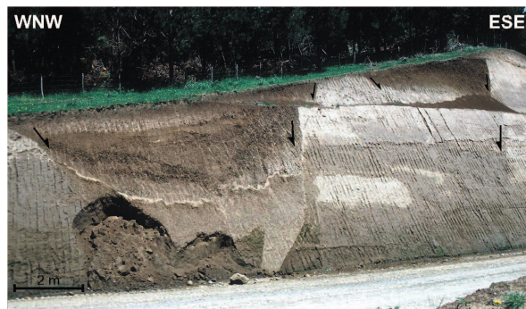
Figure 3.5: Small-scaled, NNW-SSE striking normal faults in Quaternary sediments in the Coastal Cordillera (for location see Fig. 3.1).
