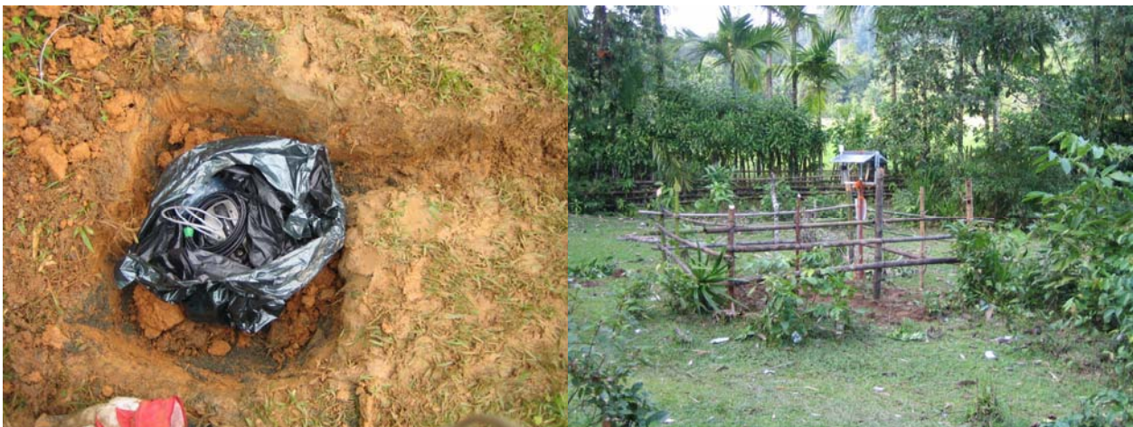
Fig. 7.5.2.1: Sensor pit and drainage channel at LABU (left). Solar panel pole and protective fence at DEHI (right).
