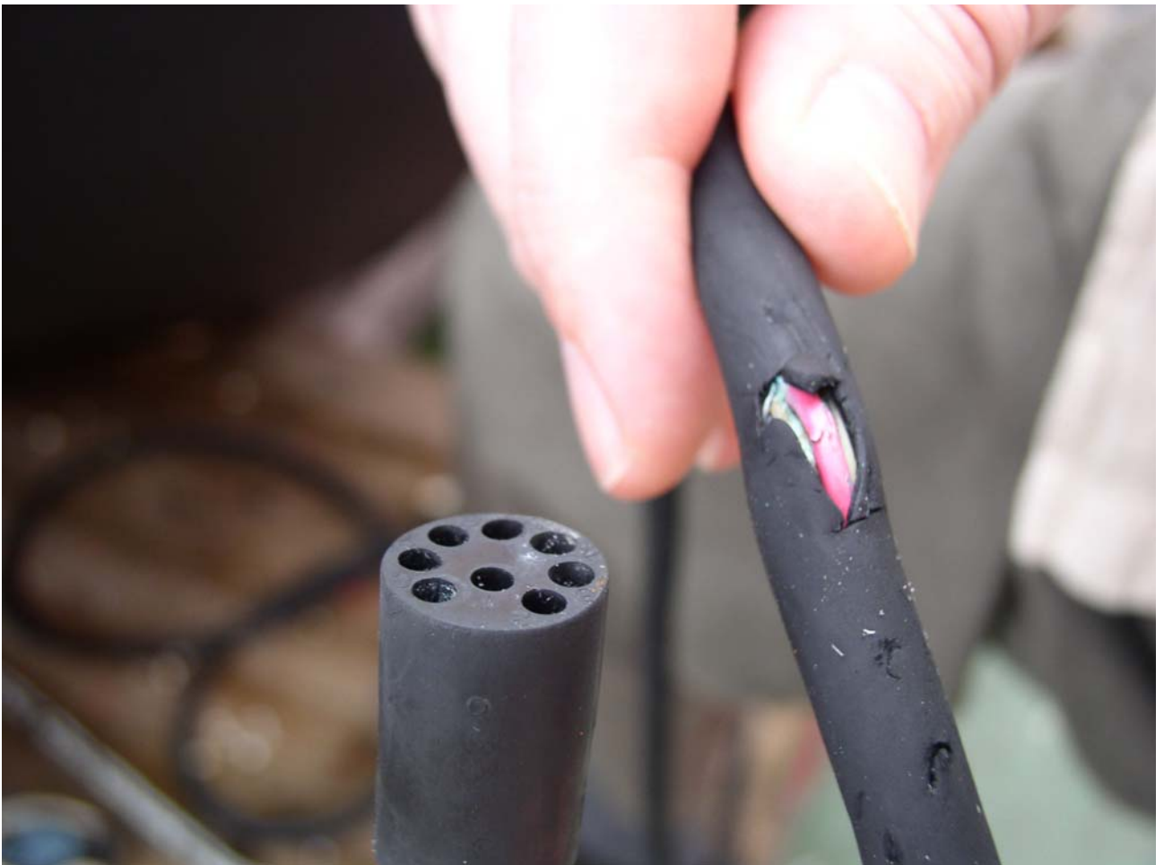
Fig. 7.6.19: Damaged cables and UW connectors after recovery
