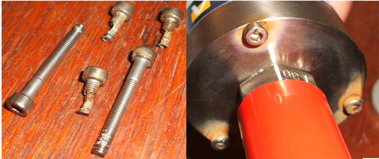
Fig. 7.5.3.1: Strongly corroded methane sensor T30, mounted on OBM02.
