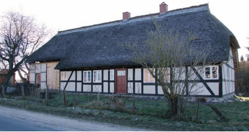
Restaurierte Querdielenbüdnerie in Below Renovated smallholding (Büdnerie) in Below with lateral entrance hall
