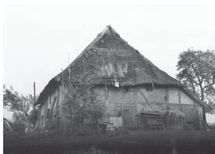
Fast verfallene Scheune und Stall Schmiedestr. 4 (1968) Mostly dilapidated barn and livestock Schmiedestr. 4 (1968)
