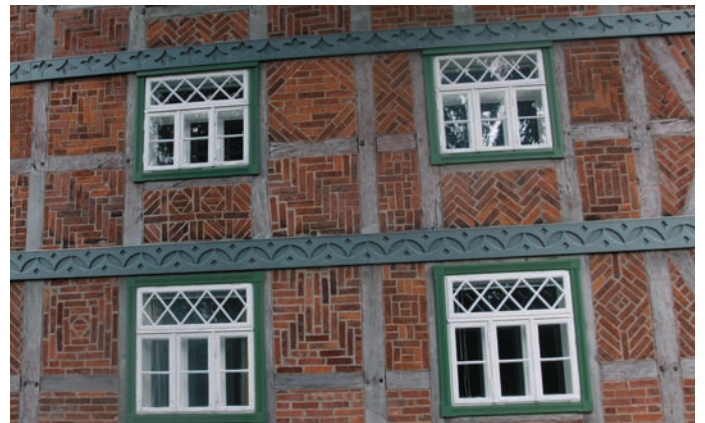
Zierausfachungen des Samenhauses in Dobbartin Ornamental breasting boards at seed store building at Dobbartin
