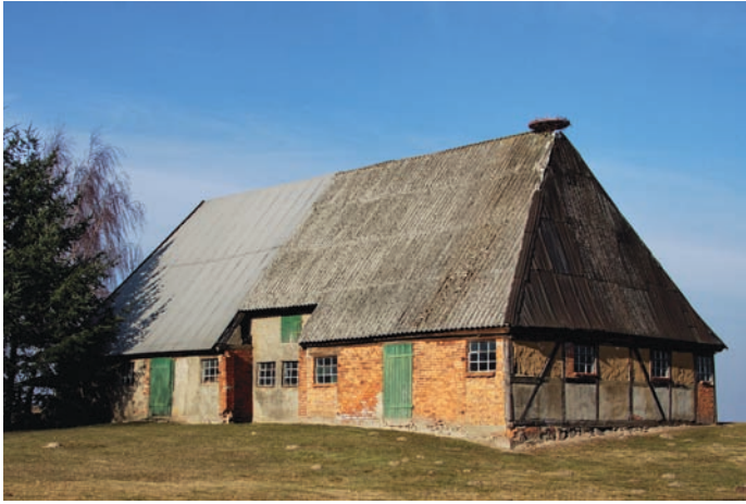
Stallscheune des ehemaligen Bauerngehöftes Hollandende 18 Livestock building plus barn of former farmstead Hollandende 18
