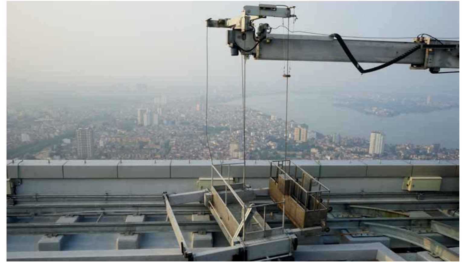
Figure 7.4. A building maintenance unit (BMU) with trolley on rail track on top of LOTTE Tower, Hanoi (Source: Michael Waibel, 2014)
