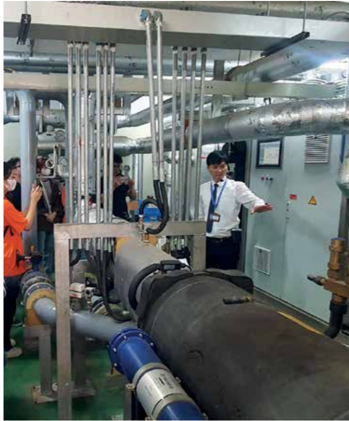
Figure 7.3. Building Technical Room at College of Urban Works Construction, Hanoi (Source: Department of Environmental Architecture, 2023)
