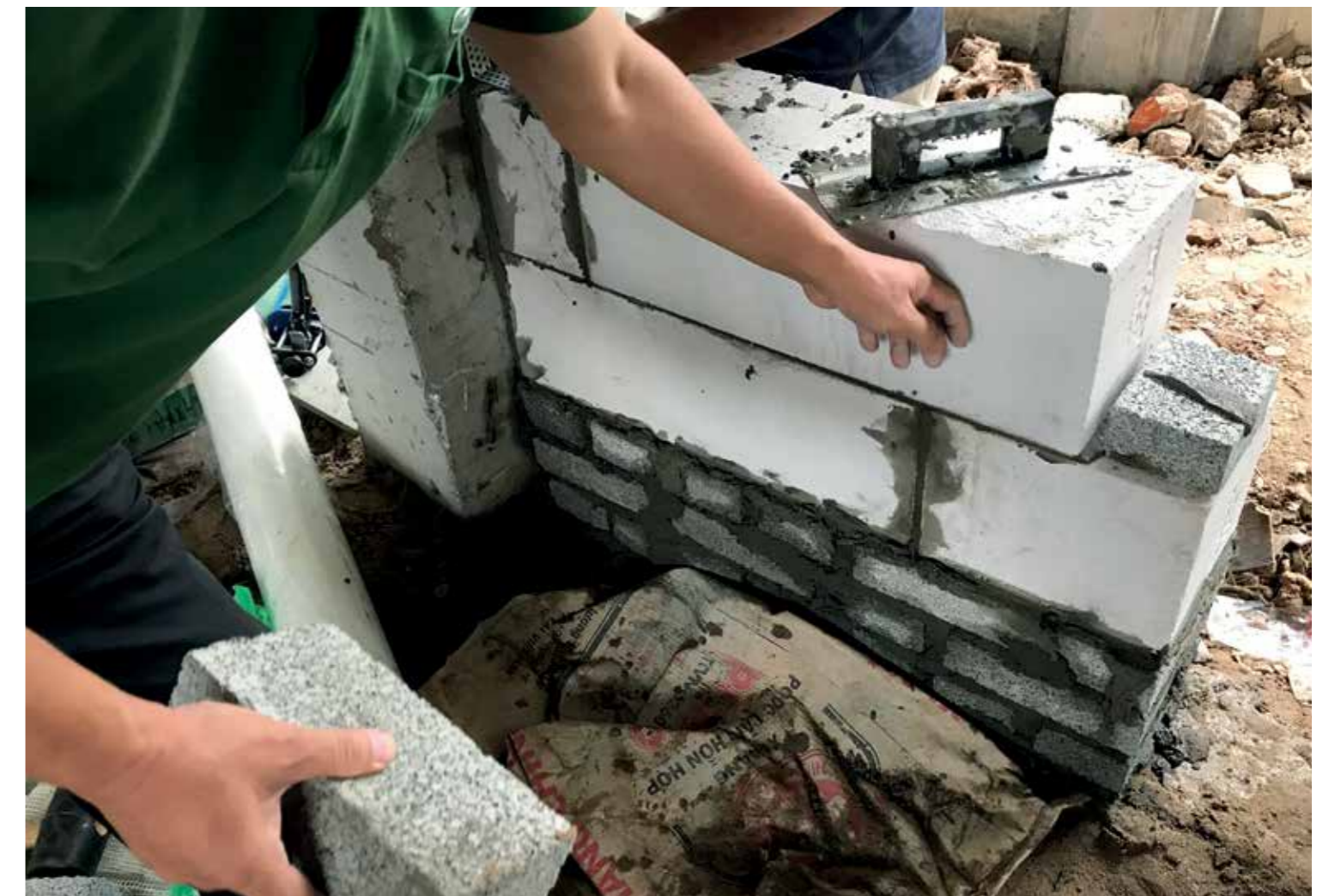
Figure 6.1. Construction of a laboratory building at Vietnam Institute for Building Materials (VIBM) in Hanoi (Source: Andreas Zegowitz)
