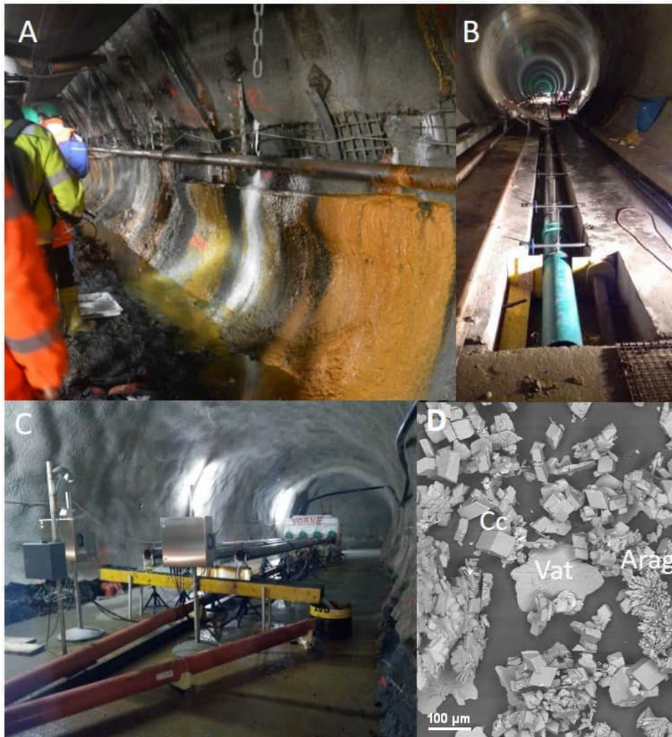
Figure 1. Diverse mineral precipitates (A) in the course of continuous groundwater discharge underground can block a tunnel drainage system (B) and were investigated by in-situ field tests (C) targeting an increased process understanding of the precipitation conditions (e.g. D: \text{CaCO}_3 polymorphism) as well as efficient countermeasures (e.g. optimized drainage design, addition of inhibitors).
