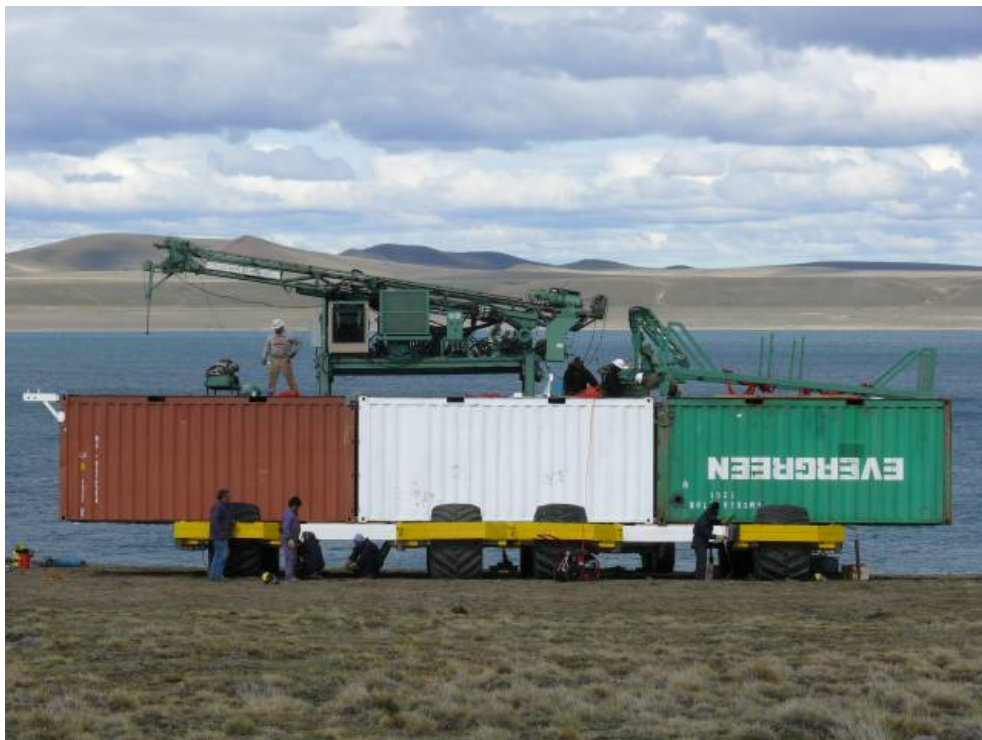
Fig. 4: The “launcher” transporting the platform and the drill rig down the lake shore and into the lake.
