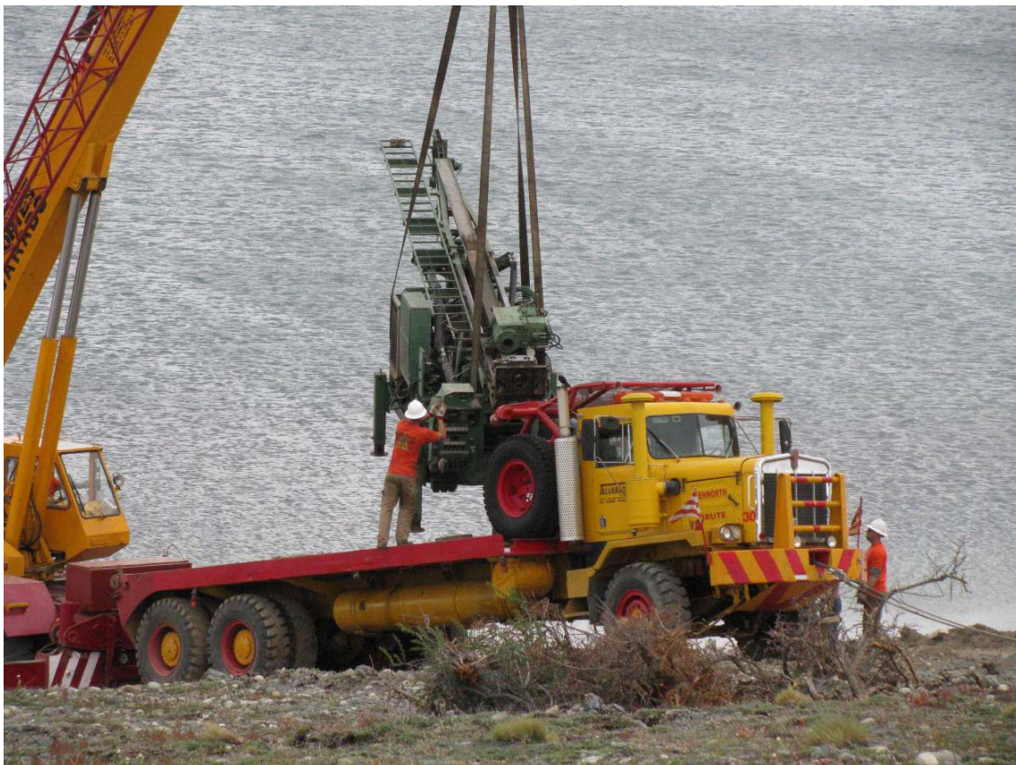
Fig. 17: Crane truck at the lake shore lifting the drill rig onto the flatboard of one of the oilfield trucks during demobilisation.
