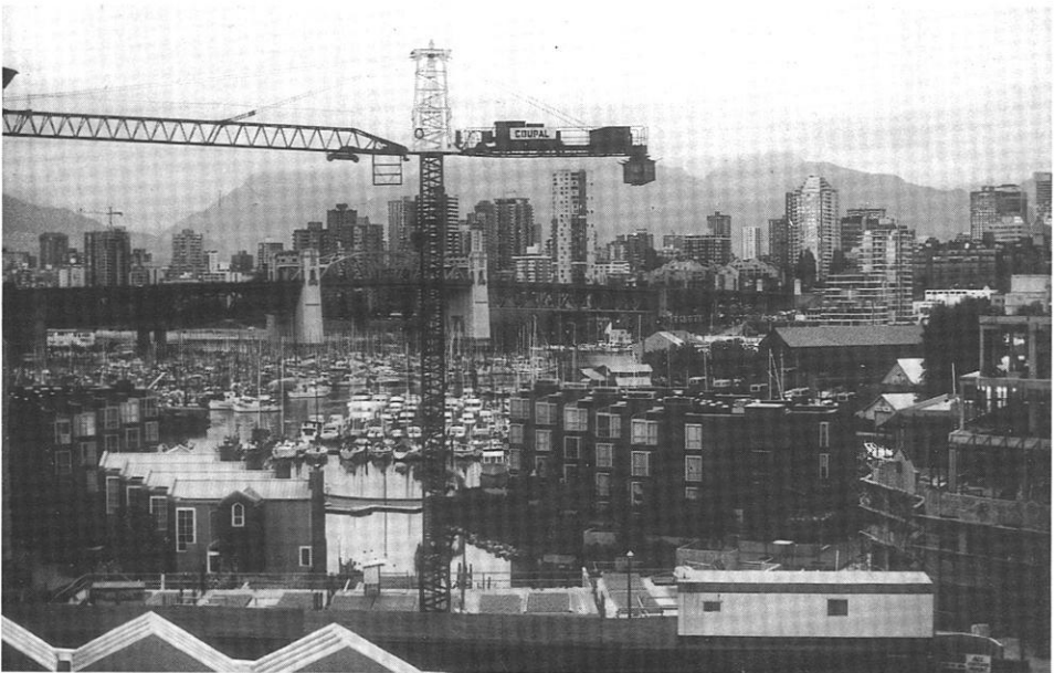
Photo 9: View northwards of False Creek, including Granville Island and downtown residential towers. Aug. 1988
