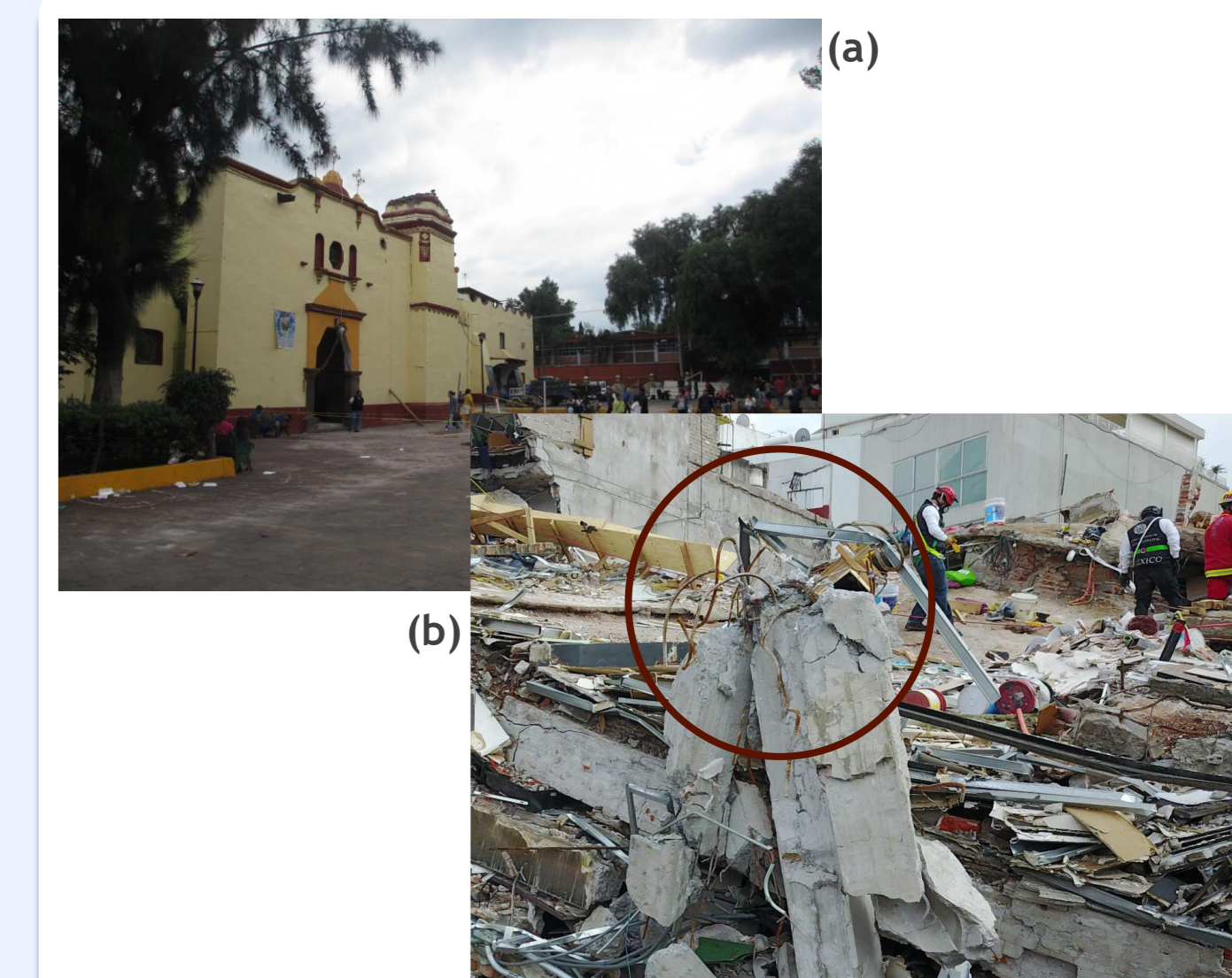
Fig. 7. Damages after the 19.09.2017. (a) Several old churches had severe damages. (b) Damages due to bad quality in buildings materials and construction.
