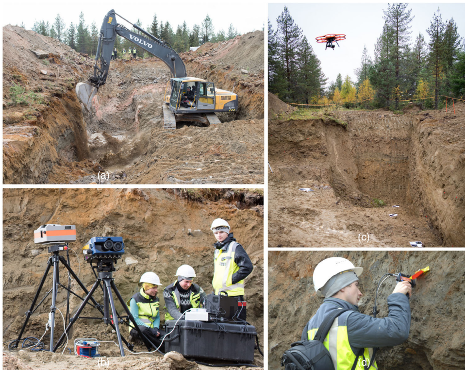
FIG. 3. Field logistics involving: (a) excavation of the trench; (b) ground-based hyperspectral imaging using an Aisa FENIX VNIR-SWIR camera; (c) UAV-based photogrammetric survey of the trenches; and (d) field validation (sampling and measurements) using handheld analytical devices (a portable VNIR-SWIR spectrometer is shown).
