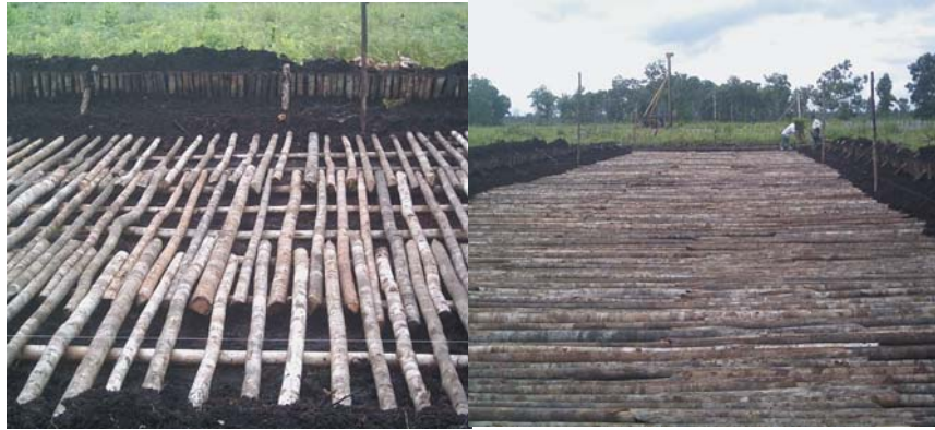
Fig. 1-3. Wooden Raft Foundation: piles laid down alternately (left), piles laid down closely (right)
