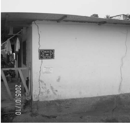
Figure 3: Fissurations of the houses.
