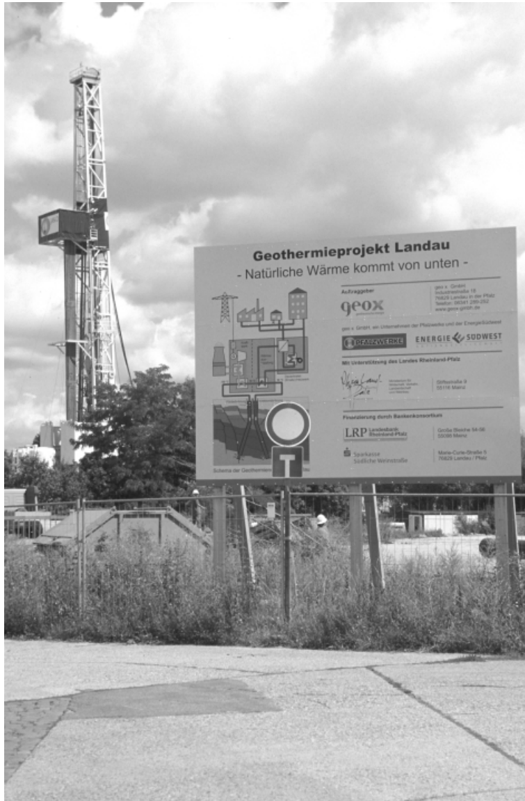
Abb. 10: Tiefbohrung, Geothermieprojekt Landau 2005 (Oil & Gas Exploration Company Jasto Ltd.; Foto: W. KUHN, LGB).
