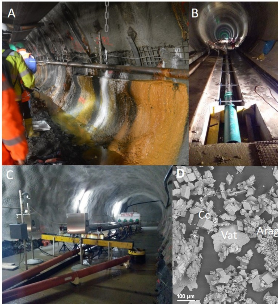
Figure 1. Diverse mineral precipitates (A) in the course of continuous groundwater discharge underground can block a tunnel drainage system (B) and were investigated by in-situ field tests (C) targeting an increased process understanding of the precipitation conditions (e.g. D: \text{CaCO}_3 polymorphism) as well as efficient countermeasures (e.g. optimized drainage design, addition of inhibitors).
