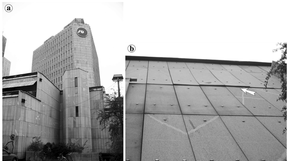
Fig. 1 Cezlak Granodiorite: a used as panels (size of slabs: mainly 1,700 × 375 × 20 mm, Maxi-Market, Ljubljana). b Detail of a W-facade showing clearly the phenomena of bowing. The texture of the rock was not considered during cutting process
